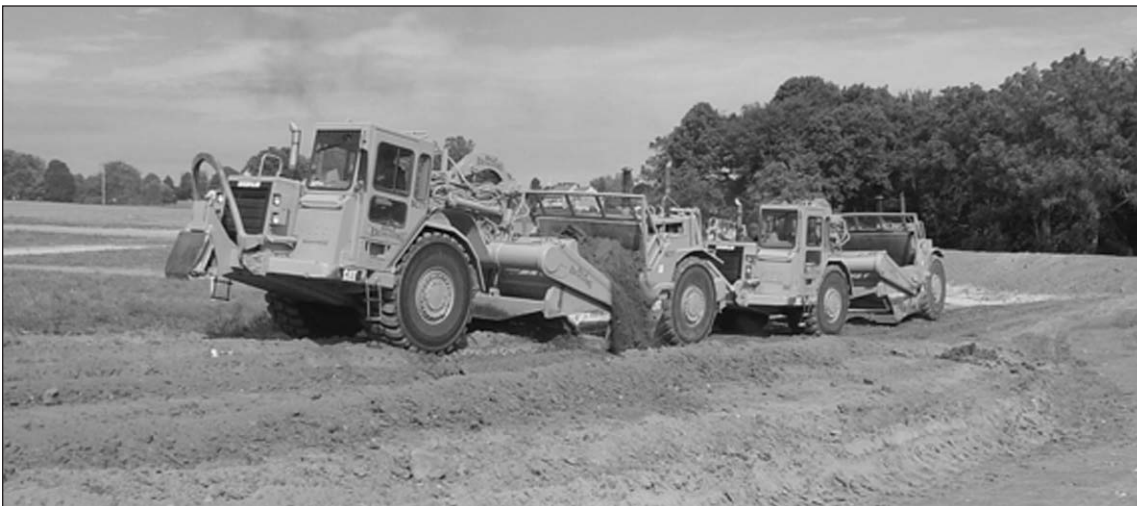
Two pans work in tandem to remove the topsoil for later use. Photo taken on Saturday, September 24, 2005
